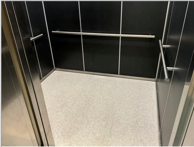
LOBBY LOOKING AT CABS (WITH DOORS OPEN)
