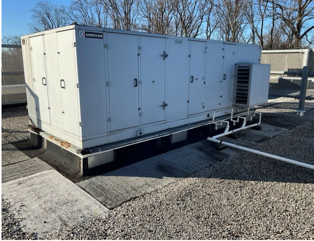
19 - ROOFTOP MECHANICAL EQUIPMENT
