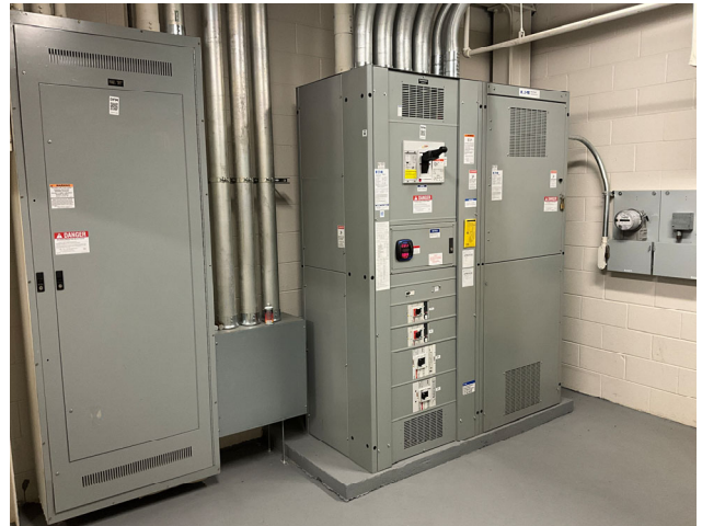
22 - MAIN ELECTRICAL ROOM
