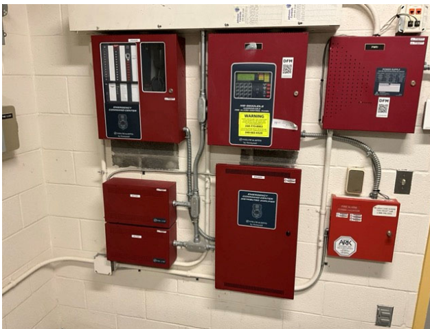
23 - FIRE ALARM PANEL
