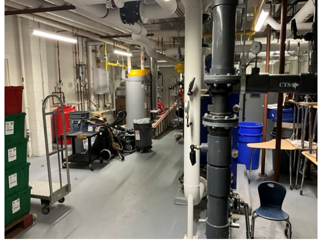
20 - MAIN MECHANICAL ROOM
